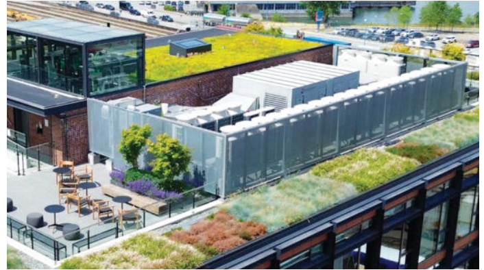
Figure 31 - Ensure exterior mechanical equipment is well integrated and screened with high quality materials. Source: ZinCo. Roof Garden. https://www.zinco.ca/intensive-roof-garden
